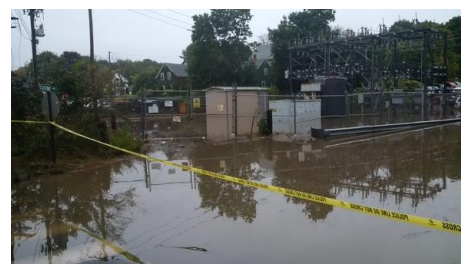
Flooded substation in Bath, Maine. Source: Central Maine Power
